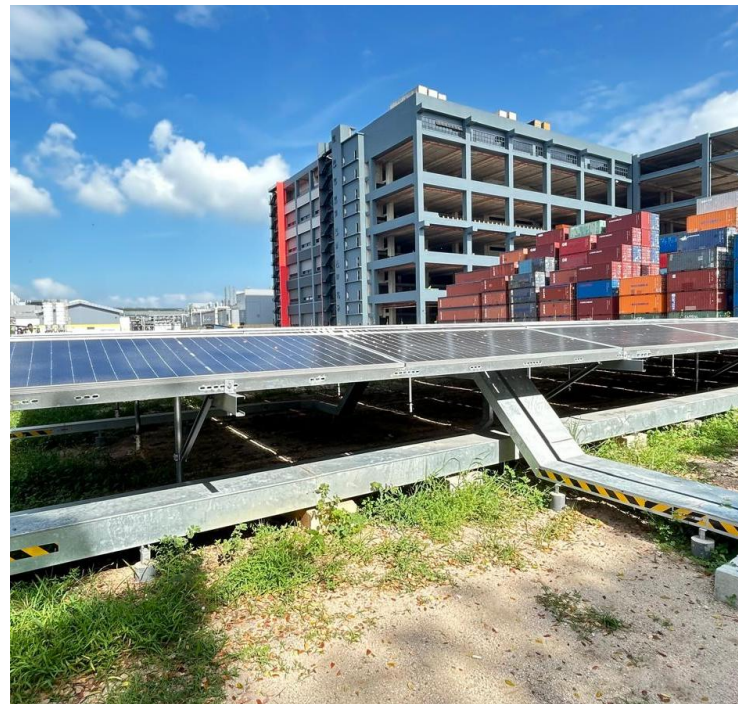
Solarland @ Tuas South
