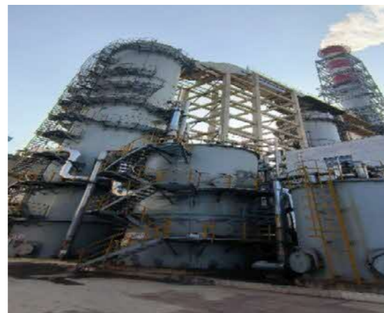
System Upgrades to Control Ammonia Escape
