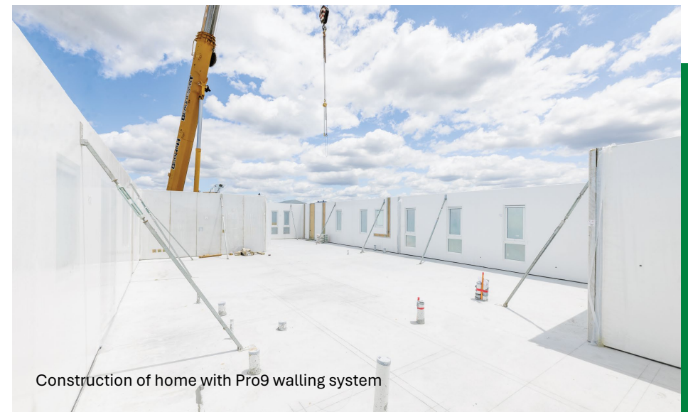
Pro9 walling being installed for a Stellar Collection home at Riverton, Jimboomba
