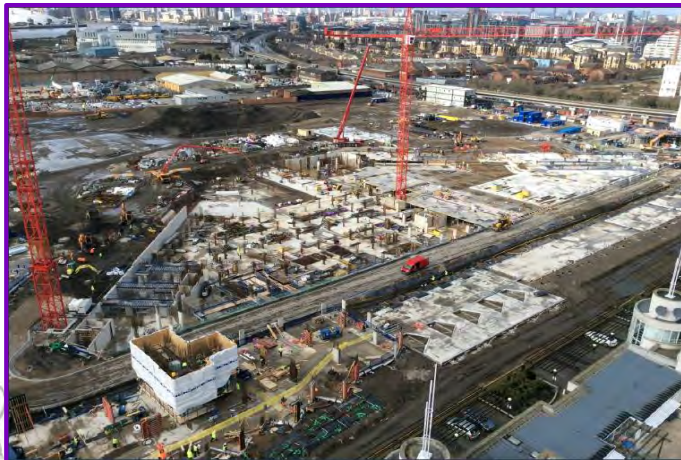
Phase 1 - Basement slabs at Admiralty and Maritime Building almost complete as at end Feb'15
