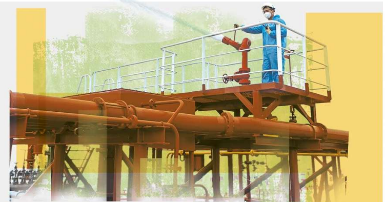
Fire Fighting System Inspection
