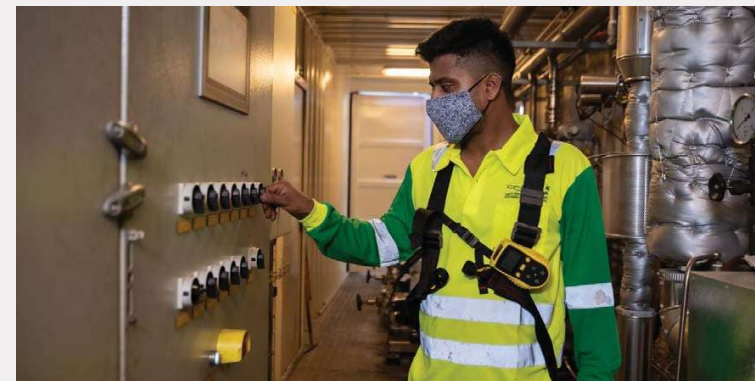
Cogent Holdings' Tank Depot Technician at Work
