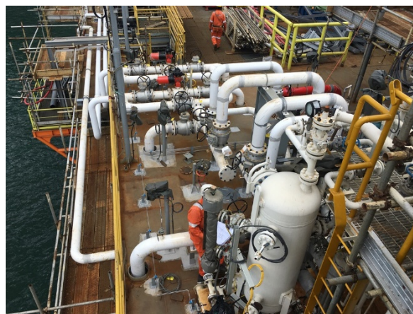
Process pipework on the deck of Ingenium II production barge
