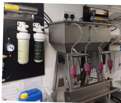
ECOPURE Water system at Crowne Plaza Nottingham
