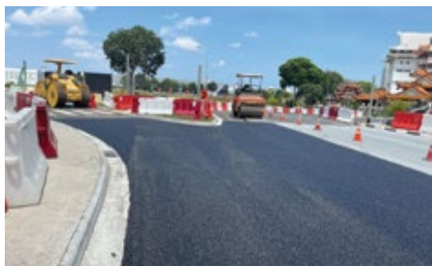
OKP is involved in the widening of Tampines Road between Kallang Paya Lebar Expressway (KPE) and Tampines Avenue 10.
