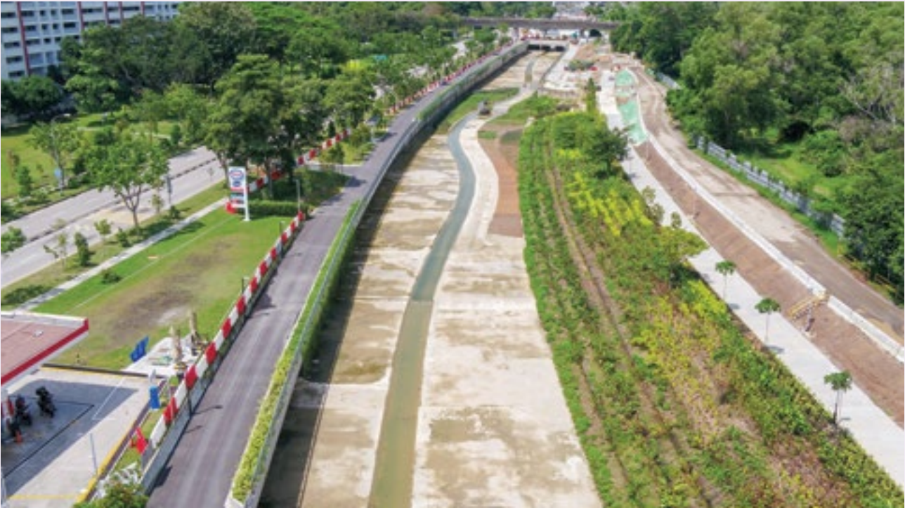
OKP is involved in the improvement to Sungei Tampines (Tampines Avenue 7 to Tampines Expressway).
