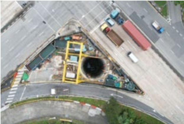
OKP is involved in the construction of link sewers from the Deep Tunnel Sewerage System phase 2 project – schedule III contract 1 (Jalan Buroh/ Tanjong Kling Road).
