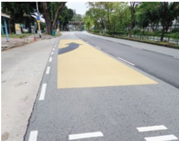
Road maintenance contract for North East Sector is one of OKP's ongoing maintenance projects.
