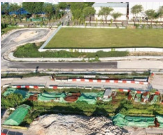
Proposed construction of new infrastructure at Tukang Estate is an ongoing OKP's construction project.
