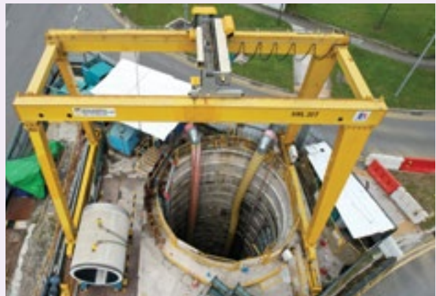
The construction of link sewers from the Deep Tunnel Sewerage System phase 2 project – schedule III contract 1 (Jalan Buroh/Tanjong Kling Road) is an ongoing project.
