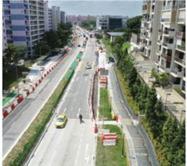
One of OKP's ongoing construction projects involves commuter and road infrastructure works in Pasir Ris and Loyang.
