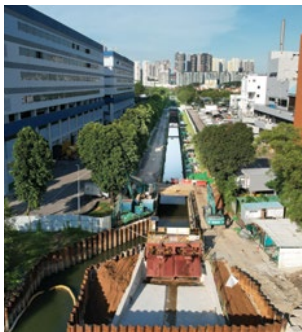
OKP is involved in the improvement of West Coast outlet drain No. 6 (after Pandan Loop to the sea).
