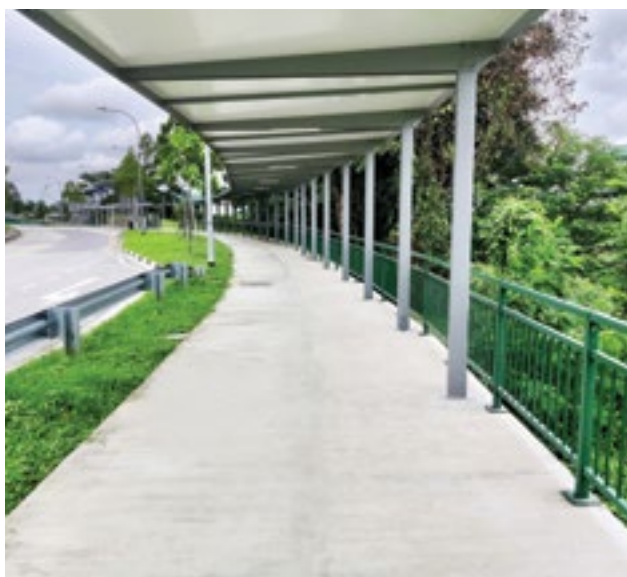
OKP is involved in the construction of covered linkways to Thomson East Coast Line (TEL) Stage 1, 2 and 3 Stations (Caldecott).
