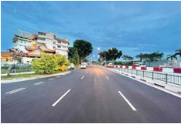
The widening of Tampines Road between Kallang Paya Lebar Expressway (KPE) and Tampines Avenue 10 is an ongoing project.
