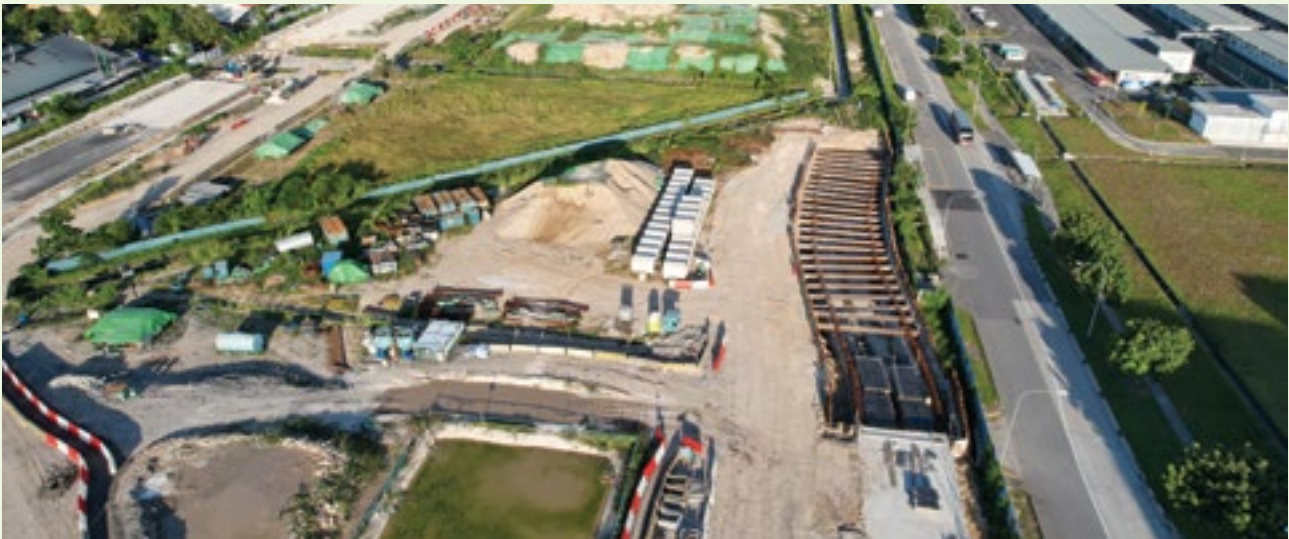
OKP is involved in the construction of new infrastructure at Tukang Estate.
