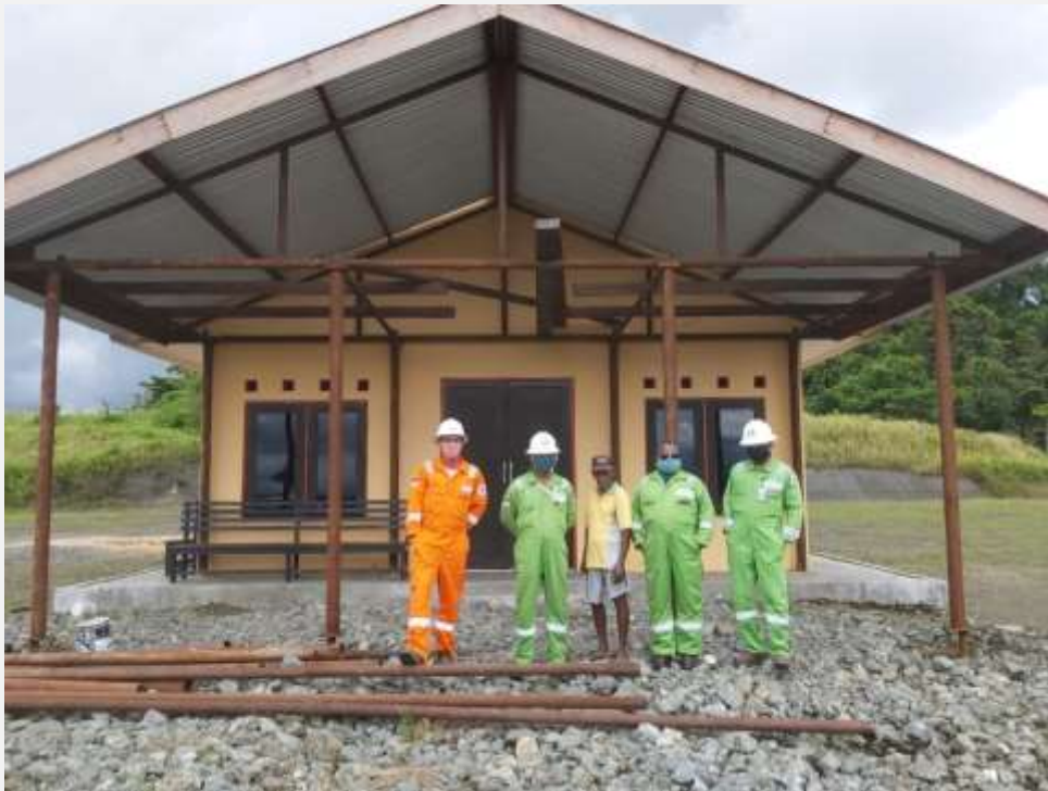
Carried out church renovation work and added church pulpit facilities for the Christian community in the Sakarum village, Seget District.
