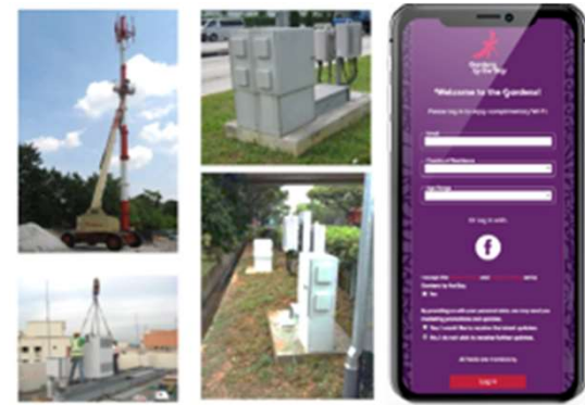
5G and WiFi infrastructure
