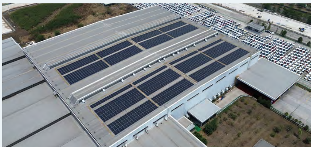
Solar panels at PT Astra Daihatsu Motor
