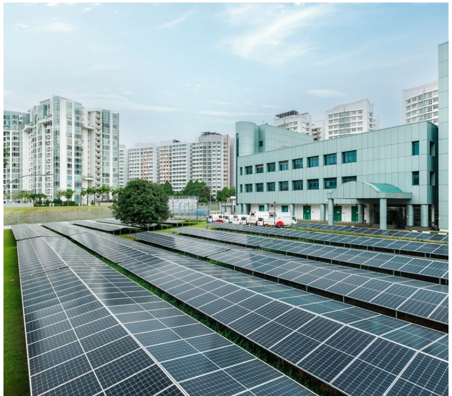
Solar photovoltaic panels at Hougang Telephone Exchange.
