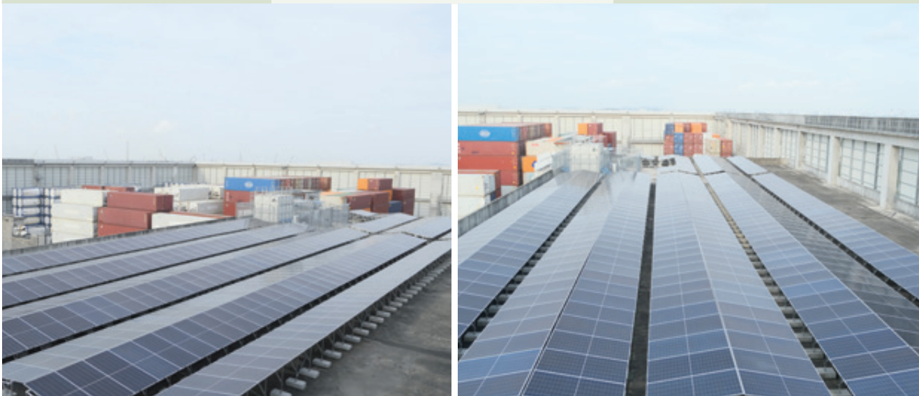
Photographs taken at the Jurong Island Logistics Hub PV system
