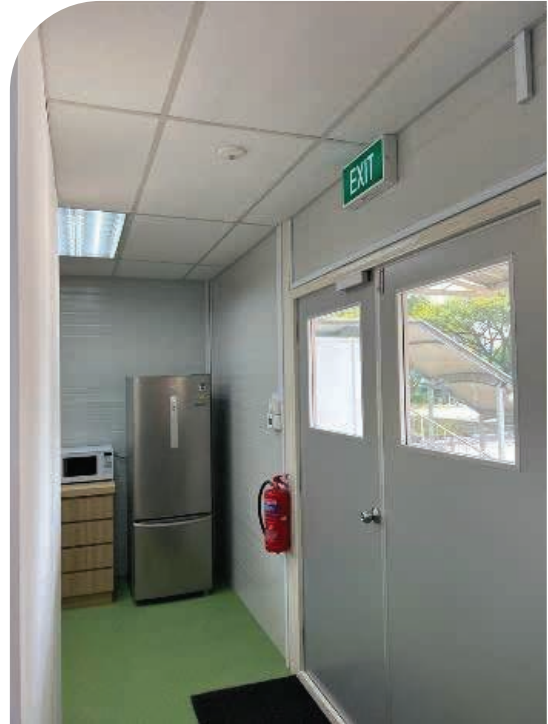
Motion sensor at office entrance
