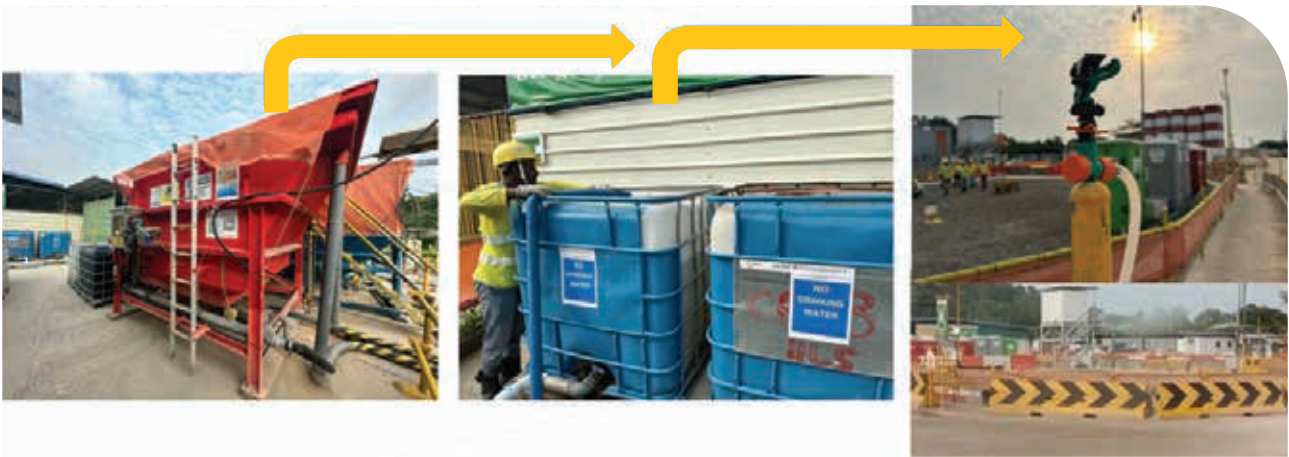
Recycled water from ECM (erosion control measure) tank used for dust control.
