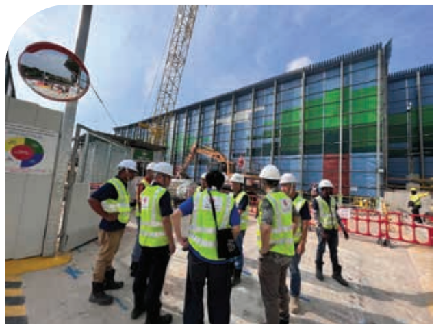
Board Independent Directors visited Serangoon North MRT Station construction site on 12 October 2023 to promote safety awareness
