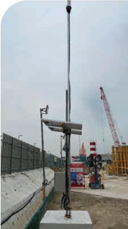
Solar panel for powering up CCTV
