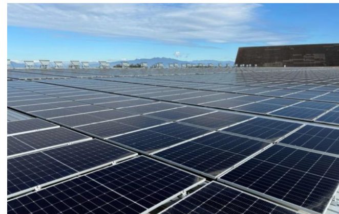
Solar panels installed on the rooftop of DPL Gunma Fujioka
