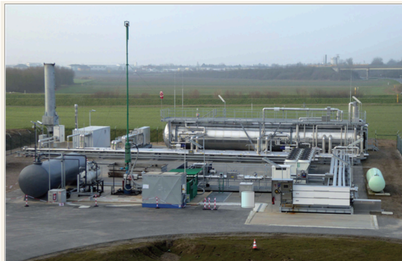
Fig. 4.4 Schwarzbach processing facility
