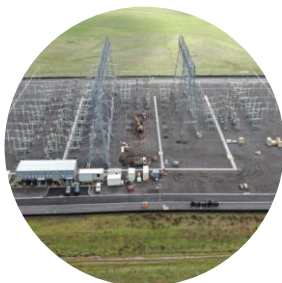
336MW Dundonnell Wind Farm FY20 forecast completion
