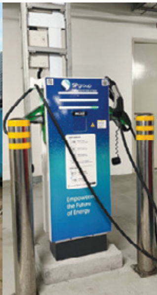
▲ EV Charging station at Paya Lebar Square
