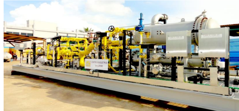
Chemical Injection Skids
