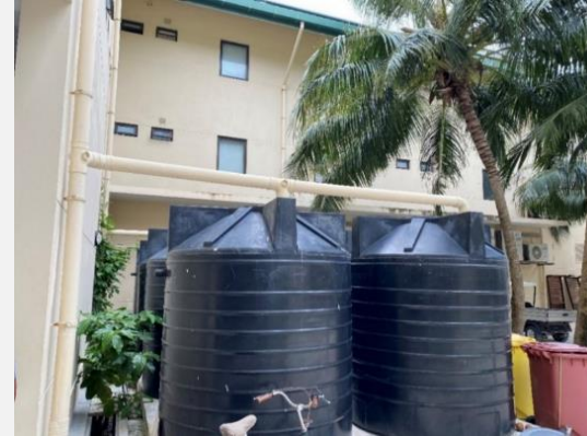
Rainwater harvesting tanks at InterContinental Maamunagau Resort
