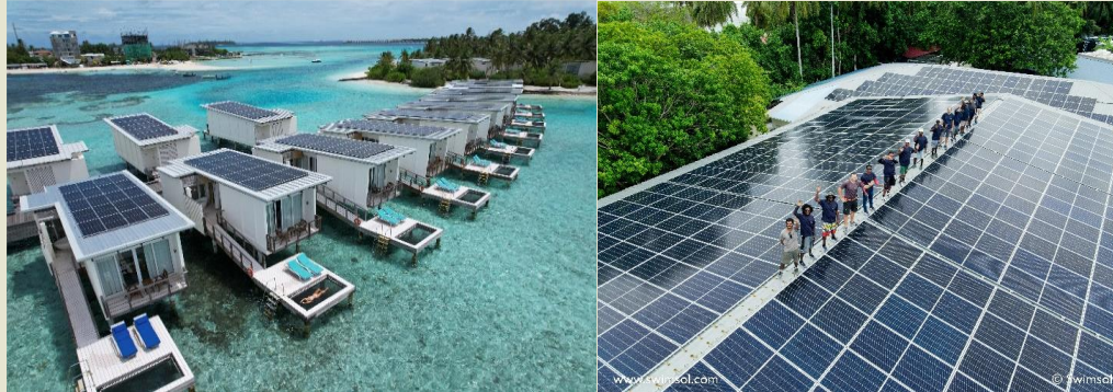
Solar Power Project at Holiday Inn Resort Kandooma Maldives
