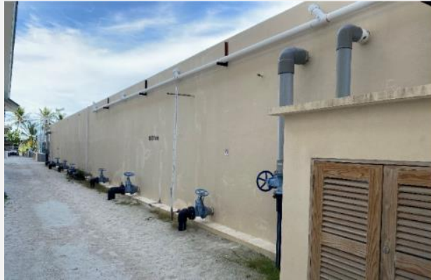
Sewage treatment plant at resort back of house
