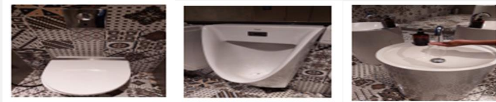
Efficient water fittings installed at Hard Rock Hotel Bali
