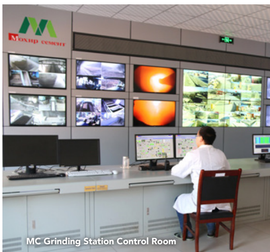
IMCCMC Cement Plant
