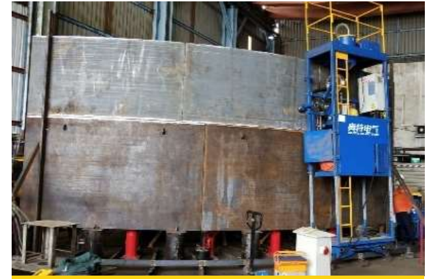
Tank Automation System
