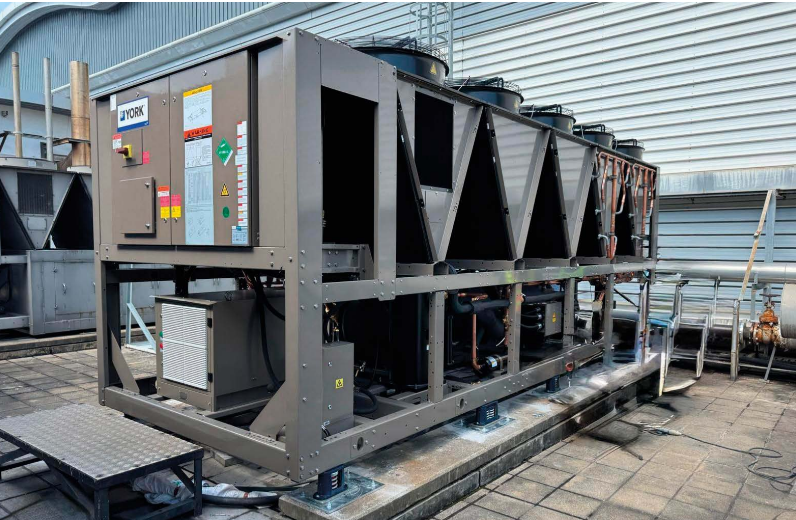
In Hong Kong, we upgraded our air-cooled chiller and transitioned to a lower GWP refrigerant, to reduce emissions.
