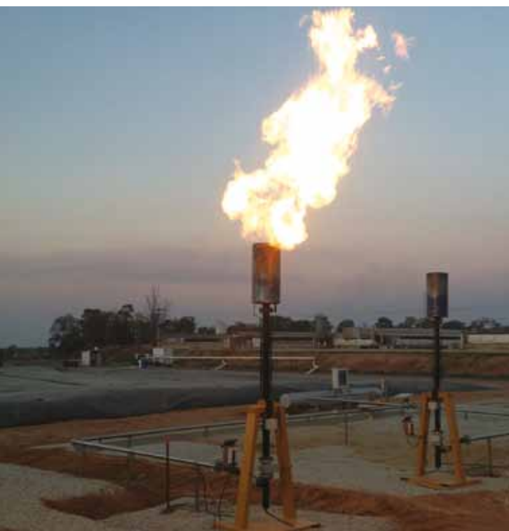
Rivalea's biogas facility
