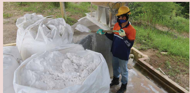
Mine effluent treatment using hydrated lime
