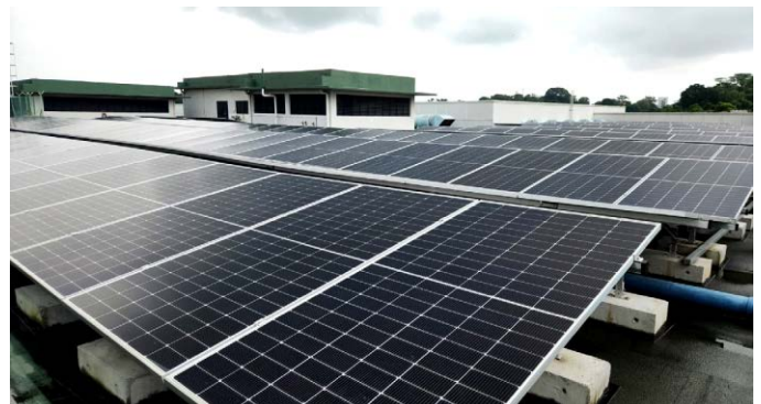
Solar panels installed at the SIA Supplies Centre
