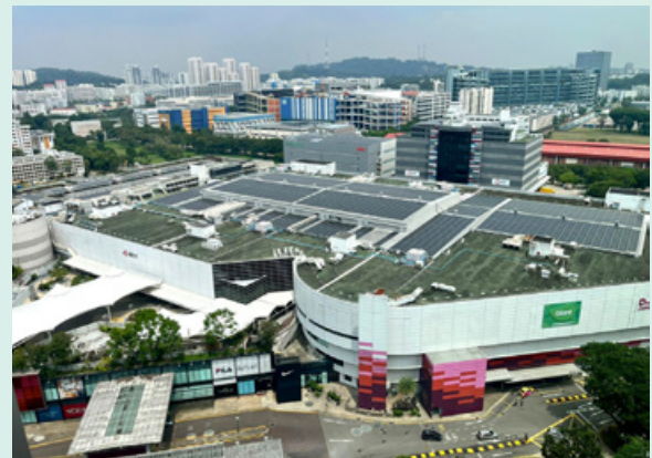
Solar panels on IMM Building's rooftop
