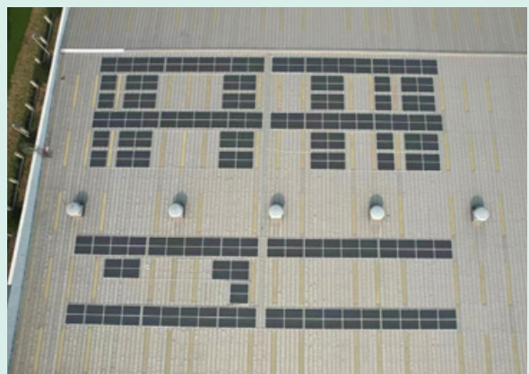
Rooftop solar panels atop Kunshan Bacheng Logistics Park
