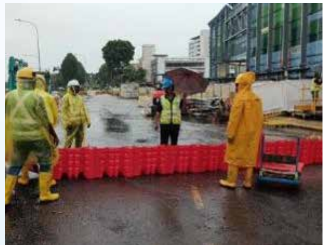
Flood barrier installed at site to divert clean water to public drains.
