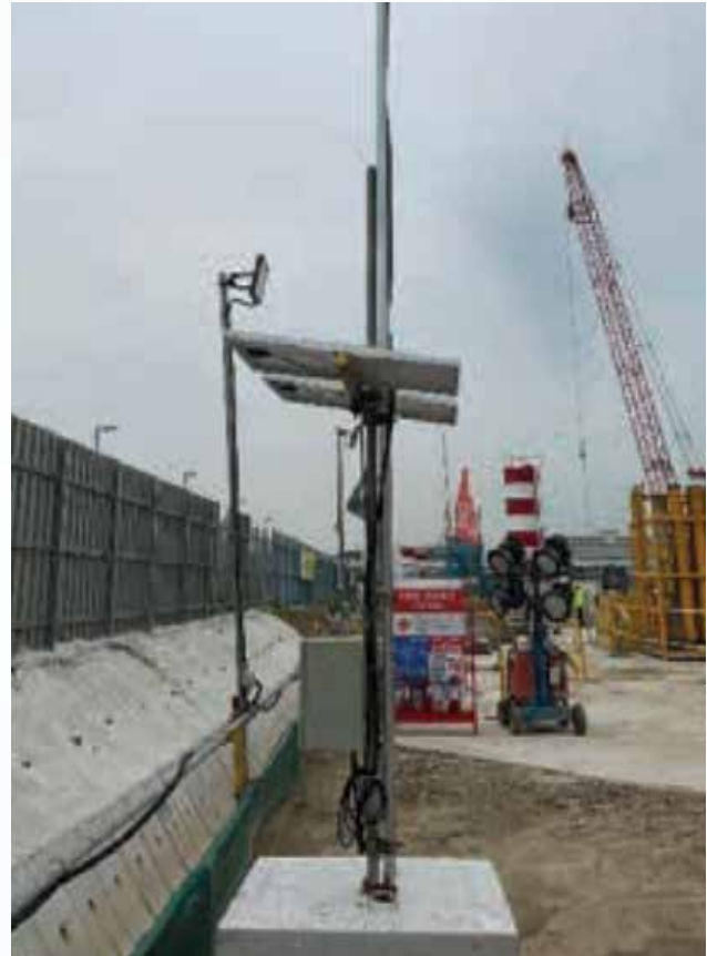
Solar panel for powering up CCTV
