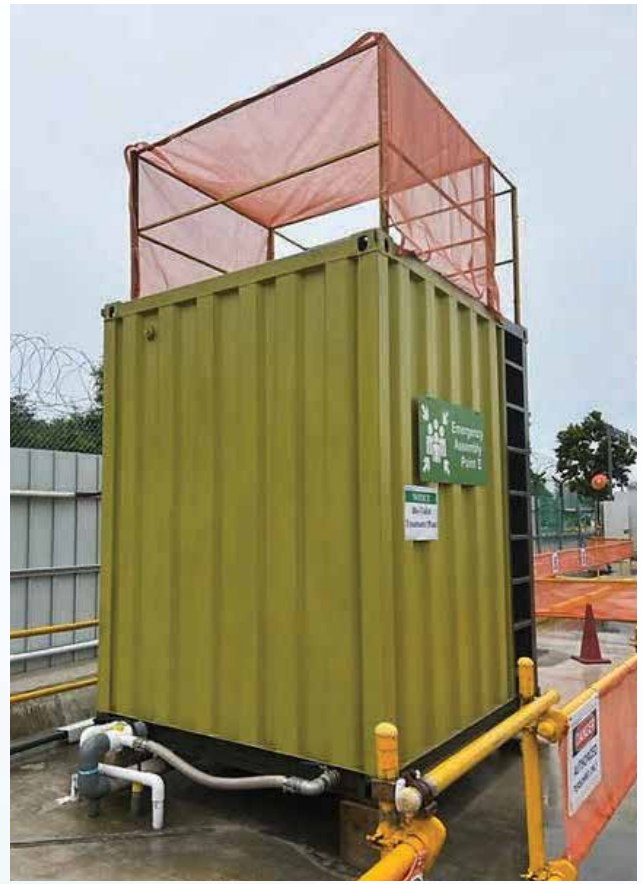
Biofuel specific membrane bio-reactor installed at a construction site.
