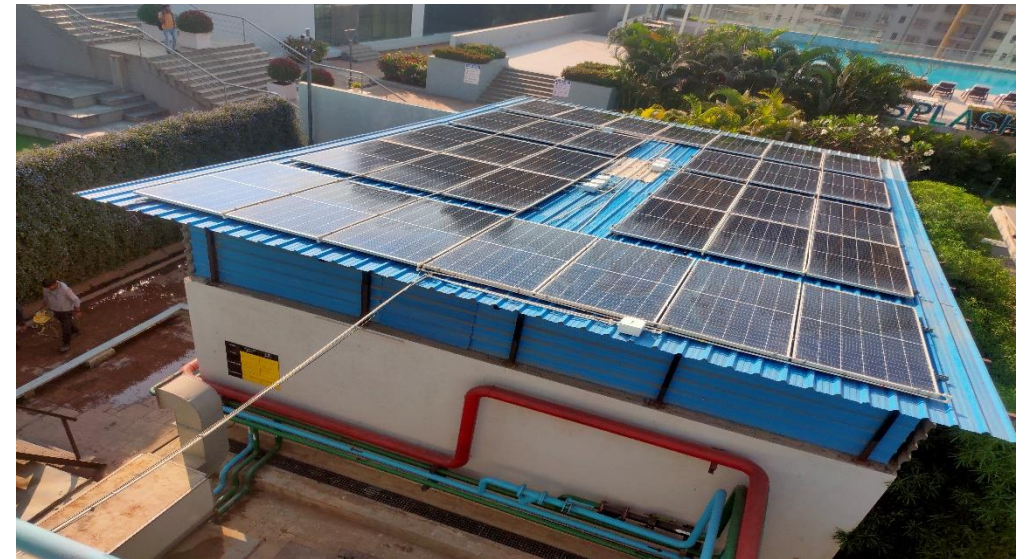
Solar Panels at aVance I, Pune
