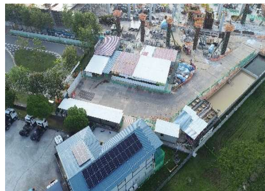
Picture 3: Solar panels installed on site office rooftop.
