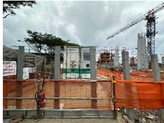
Picture 2: Battery Energy Storage System deployed at sites to reduce diesel consumption
