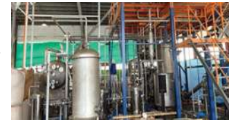
GEIH Processing facility
