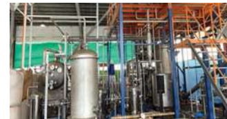
GEIH Processing facility
