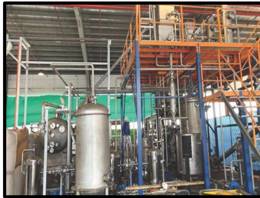
GEIH Bio-Reactor Facility : Waste + H 2 O = Steam Reforming
