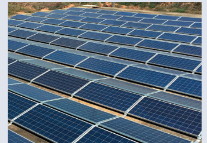
Keppel integrates its capabilities in district heating and cooling, solar energy and electric vehicle charging to offer Energy-as-a-Service, a subscription-based solution to help businesses decarbonise their operations.
