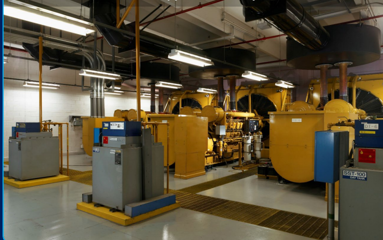
Prime-Rated Generators Support Resiliency
