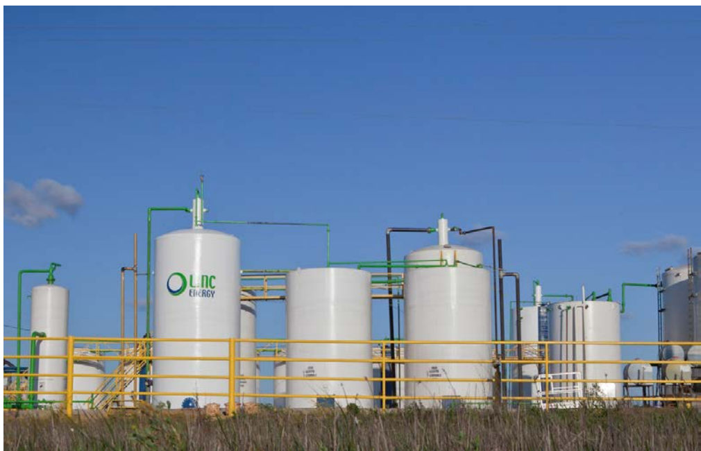
Tank batteries at Cedar Point facility
