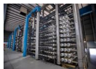
SingSpring Desalination Plant
