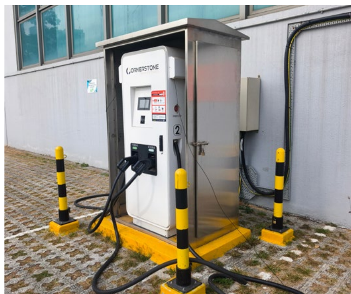
Supporting sustainable mobility at Mapletree Logistics Hub Tsing Yi with EV charging access.
