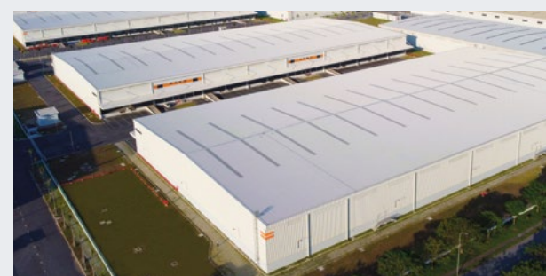
Roof reinforcement in Mapletree Logistics Park Bac Ninh Phase 4 boosts resilience against typhoons and high winds.
