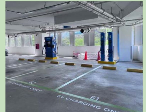
Electric vehicle charging infrastructure at 30A Kallang Place
