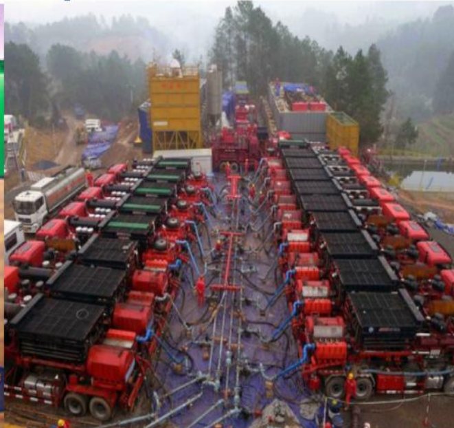
Well Engineering & optimization services
