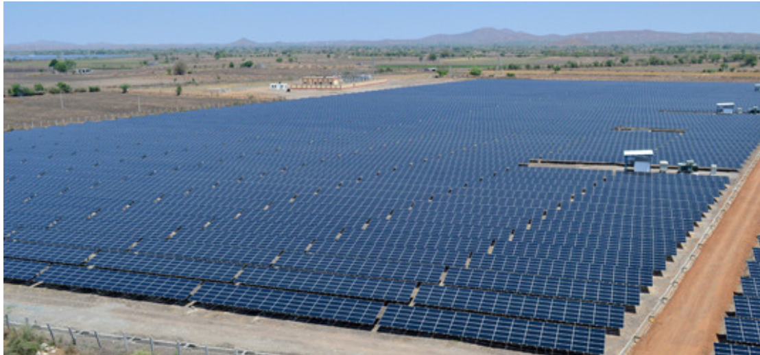
Picture: An existing 120 MW Solar PV plant in Rajasthan, India
