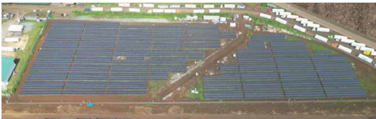
Solar energy facility located in Manolo Fortich, Bukidnon, close to manufacturing facilities
