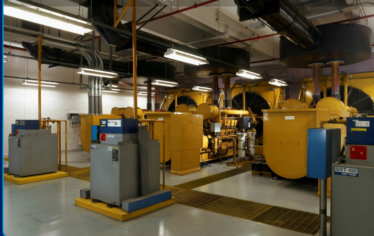
Prime-Rated Generators Support Resiliency
