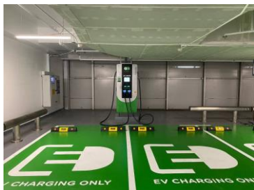
Roll out of EV car charger at Frasers Property malls
