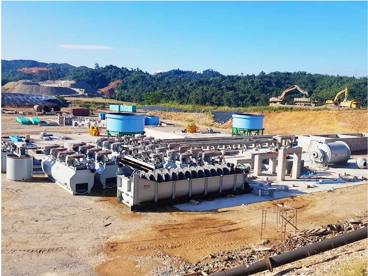
* Machineries for the proposed flotation plant at the Sokor gold field in Kelantan
