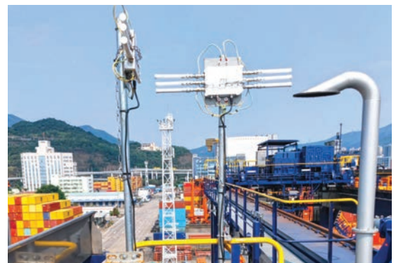
5G network technology installed at YANTIAN.
