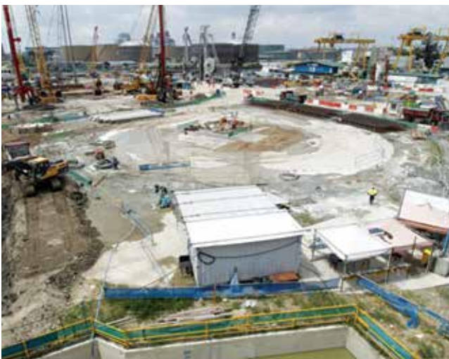
Tuas Water Reclamation Plant
