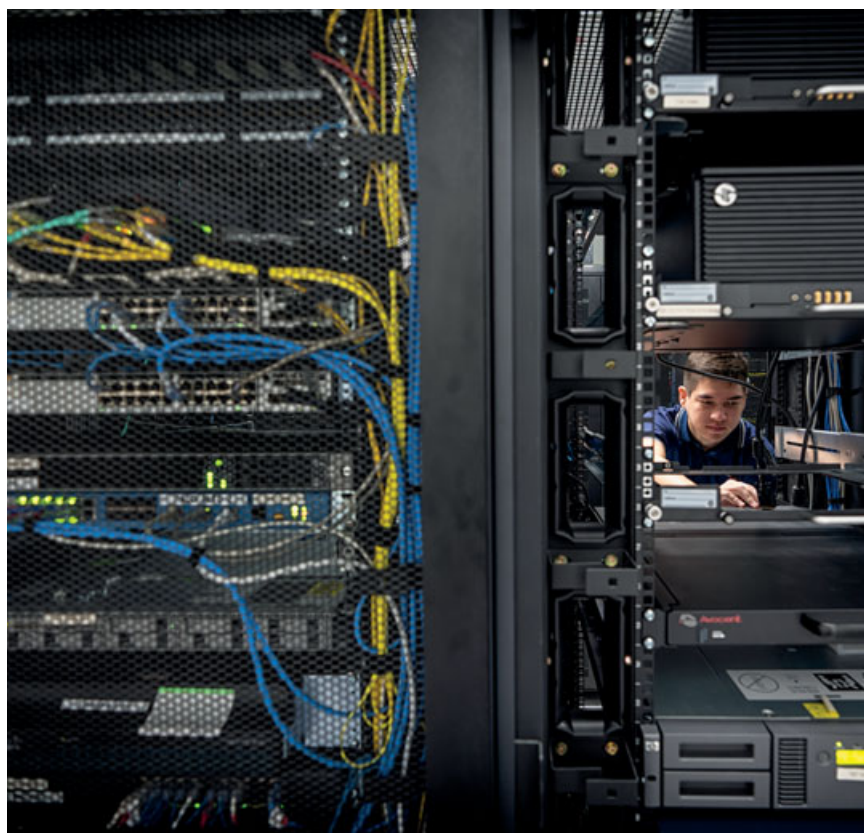
Colocation assets contributed approximately 72.4% of Keppel DC REIT's rental income.
