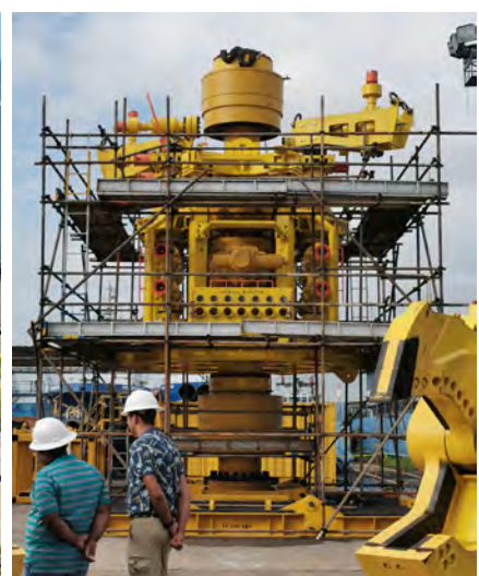
Surface Stack - Blowout Preventor commissioning
