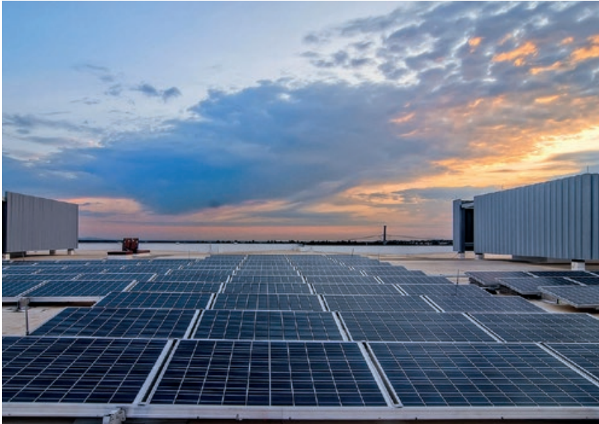
Where feasible, the Manager leverages renewable sources of energy. Pictured is an assembly of photovoltaic panels atop 105 Edgeview in Denver, Colorado.
