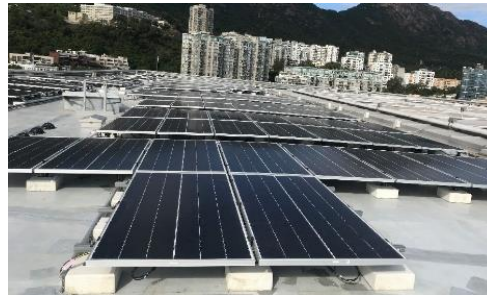
Installation of Solar Panels atop Festival Walk's office tower: These can collectively generate over 250,000 kWh of clean electricity per year.
