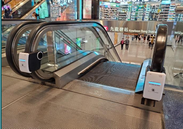
UV disinfection devices were installed on the handrails of escalators located at high traffic areas within FW
